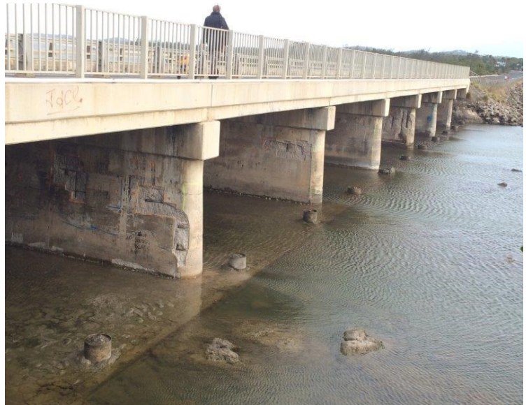
Shoal Creek Bridge at Low Tide – showing some damages
