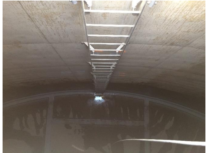
Stainless steel access ladder
