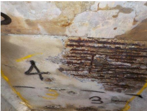
Severely damaged soffit that required extra strengthening
