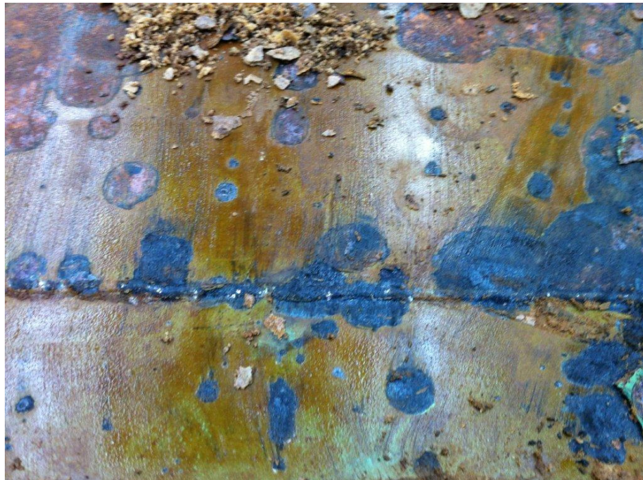
Photo showing corrosion damages to oven door
