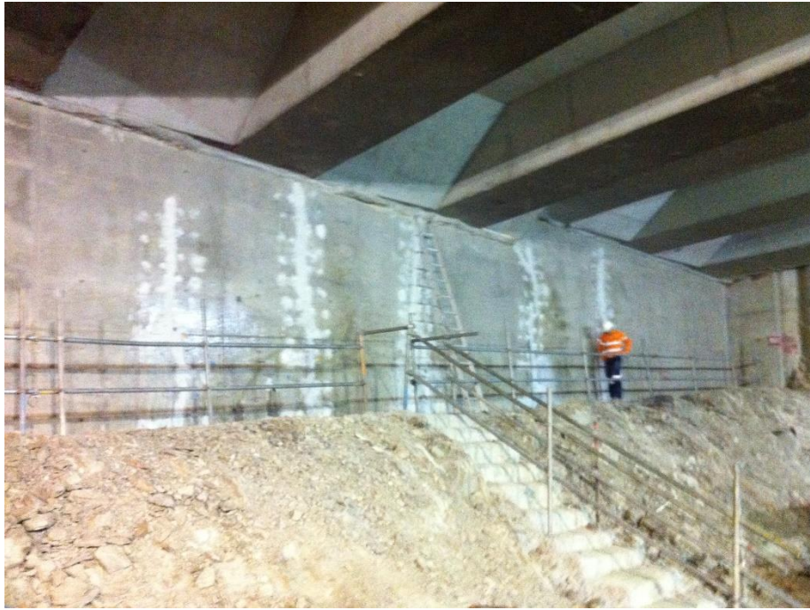
NORTH SIDE OF THE BEAM SHOWING THE FIVE CRACKS
