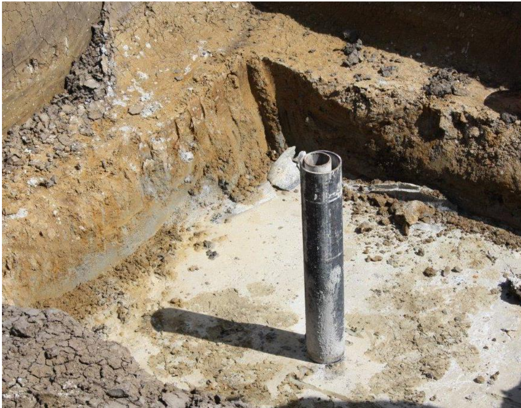
Top of the leaking gas bore
